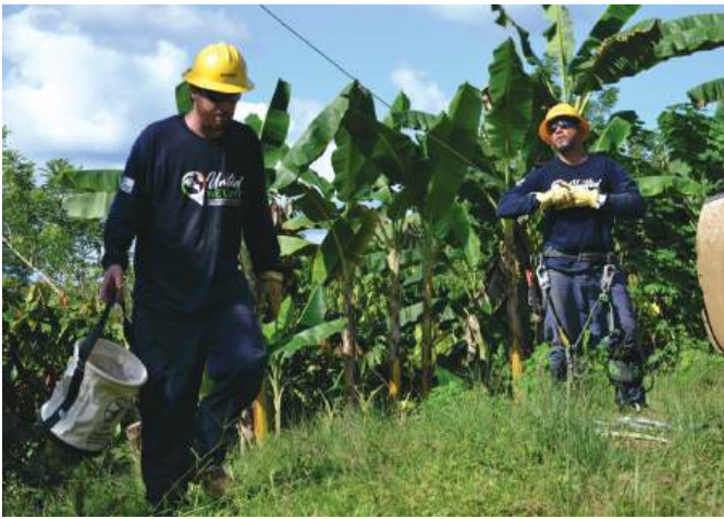
NOVEC lineworkers Blake Sparling and Mauricio Paz installed electricity for the residents of Santa Isabel, Guatemala. Photo by John Johnston.
