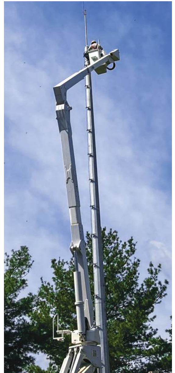
Thirty towers facilitate AMI data communications on a private network across the service territory.
